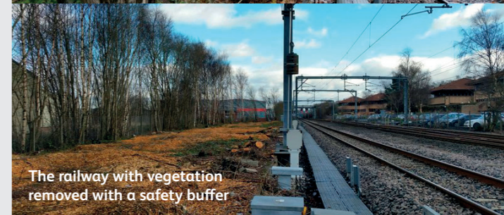
The railway with unsafe vegetation
